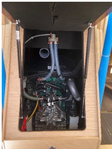
Compact – Poor ventilation
